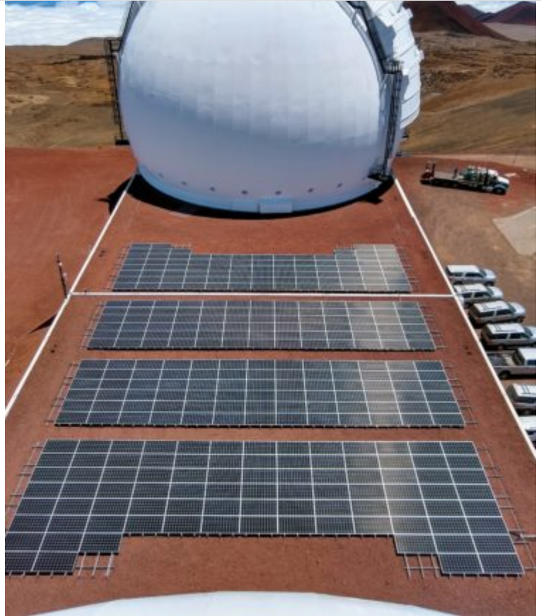
REC Solar installed a 137-kW solar system between the twin telescopes at W.M. Keck Observatory atop Maunakea, a dormant volcano and the highest point in Hawaii. Mark Devenot/W.M. Keck Observatory
