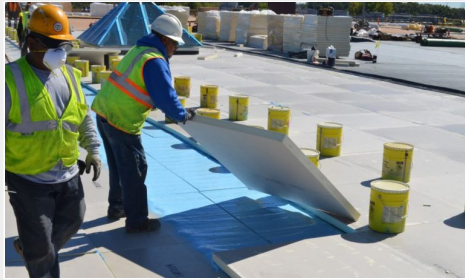
Proper installation of the insulation is key to meeting code requirements and preventing air leakage.
