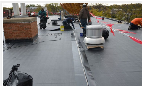
A fully-adhered membrane will prevent fluttering and minimize energy loss. Photos: Hutchinson Design Group
