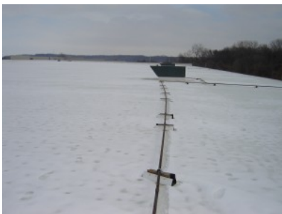
Gas lines supplying HVAC rooftop equipment can be affected by snow accumulation.
