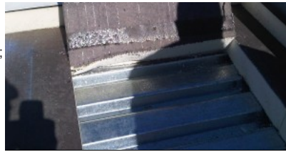
Condensation forming on the bottom of the insulation of a white roofing assembly in a northern climate.
