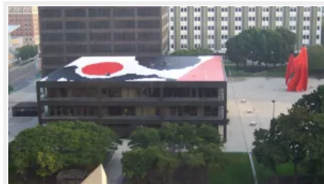
Great Lakes Systems, Jenison, Mich., was challenged to recreate the Calder mural on a new EPDM roof after tearing off the modified bitumen roof on which the mural was originally painted.
