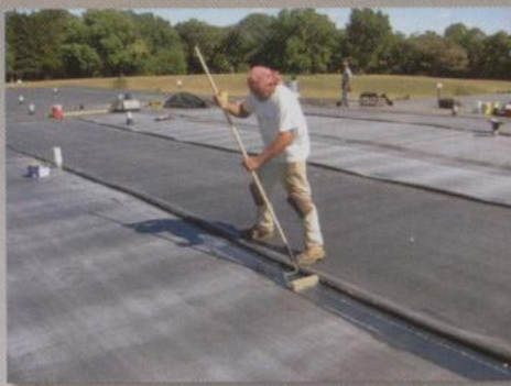
■ Proper application of the seams is a crucial component in the installation of EPDM systems. (Photo courtesy of ERA.)
