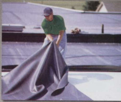
■ The EPDM Roofing Association has seen promising results in recycling programs focusing on EPDM roofs. (Photo courtesy of ERA.)
